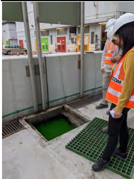
Figure.5 Dye test carried out on 30 December to ensure the gate valve is fully closed
