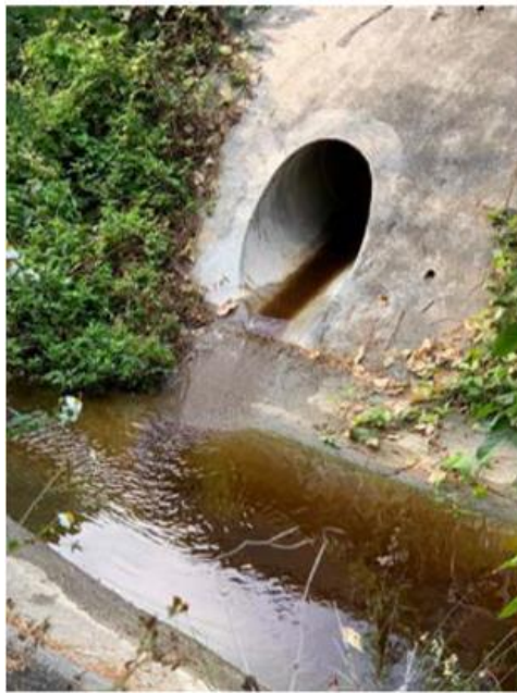
Figure.2 Clean water at the stormwater discharge outlet
