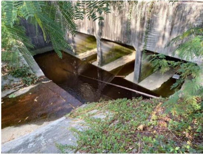
Figure.1 Slightly brown colour water at the pit of nullah
