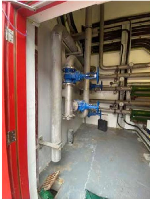
Figure.3 Misalignment of overflow pipeline to the drain pit inside the TE pump room
