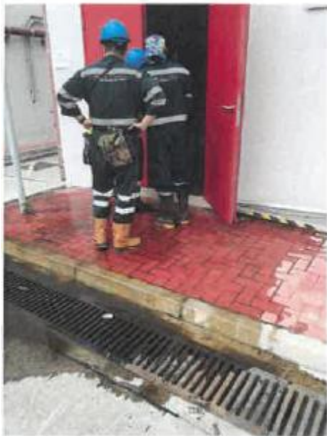
Figure.1 Brown water was found leak from treated effluent pump room
